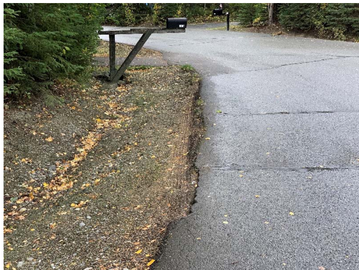
Photo 3. Pavement edge damage by traffic (mail truck)
